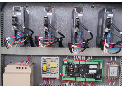
Board control system
